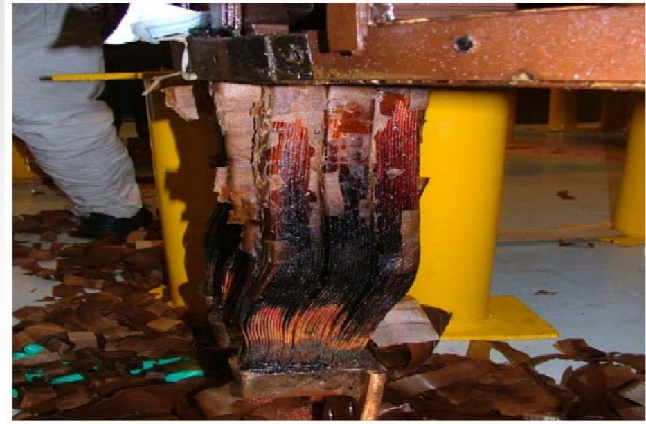
Station 3 Transformer 6 LV exit lead overheating
