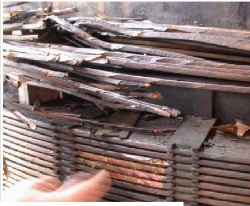
Station 4 Transformer 6 HV winding failure
